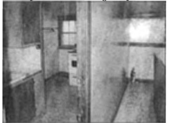
Poorly erected wall dividing third floor room:
