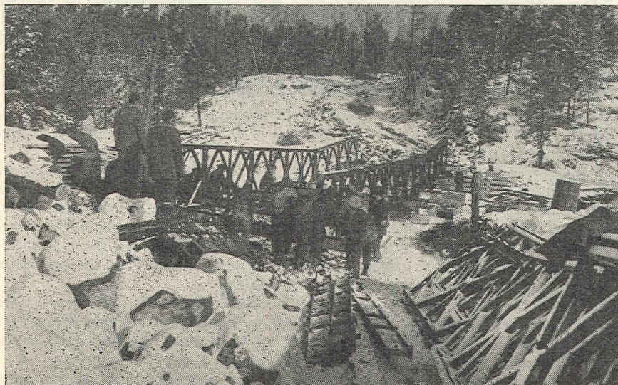
Last link in their road "outside", Dokis men finish Bailey bridge over Little French River.
